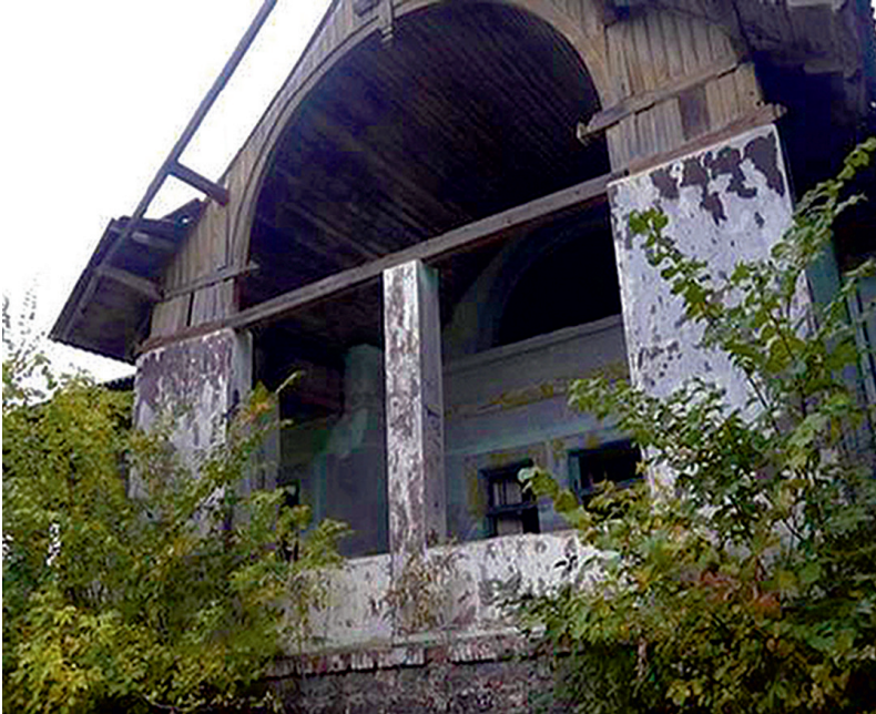
Photo 7. The disastrous state of the exterior of the Adrianovs mansion from Răspopeni village in Șoldănești district
