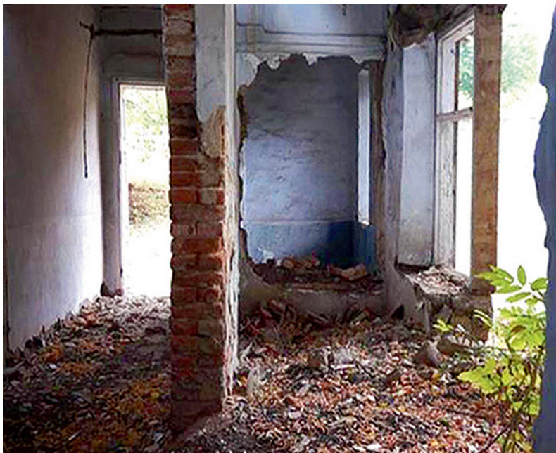
Photo 8. The internal disaster of the Adrianovs' mansion from Răspopeni village in Șoldănești district
